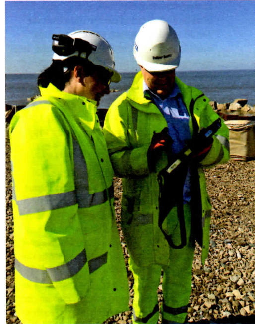
Construction team using Sitedesk on-site at Rossall Beach – Rossall Coastal Defence Scheme.
